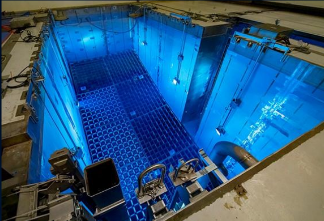
Plant Vogtle #3 Spent Fuel Pool
